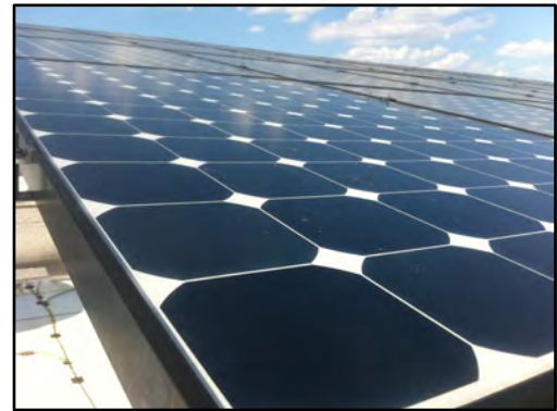
Figure 1.12. Photovoltaic array on Building 11 West Campus.
