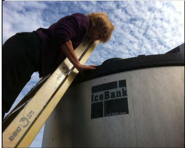
Figure 2.13. Thermal Storage Tank stores ice produced during off-peak hours to assist in cooling chilled water for use during peak hours.
